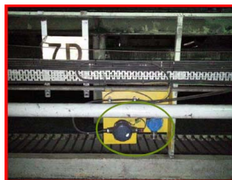
CO Sensor installed at bunker
