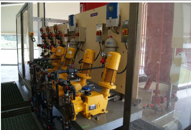
助凝劑加藥設備(助凝劑：polymer)
