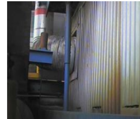
Outlet HP Superheater
