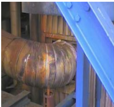
Outlet HP Evaporator
