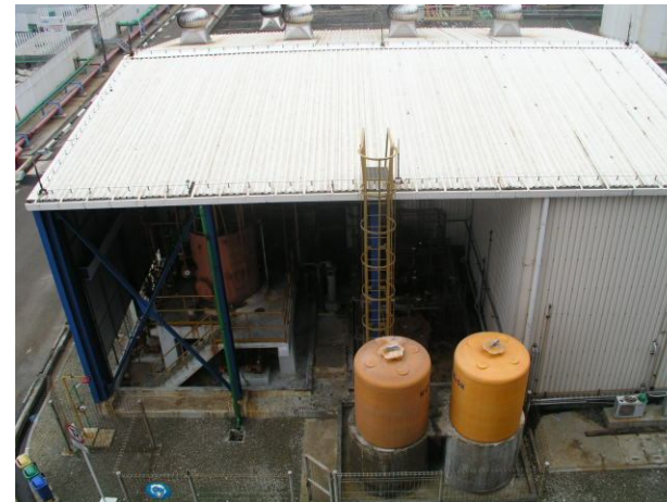
Waste Water Treatment
