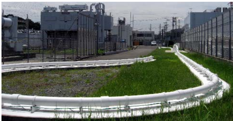
圖 10 Sumitomo 66 kV 超導電纜 at Asahi Substation, Yokohama
