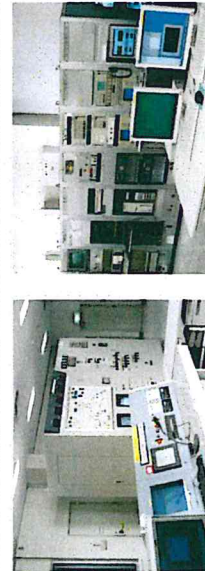
制御制御室 View of control and data acquisition section
