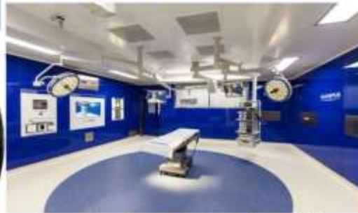
Operation Room System Integration
