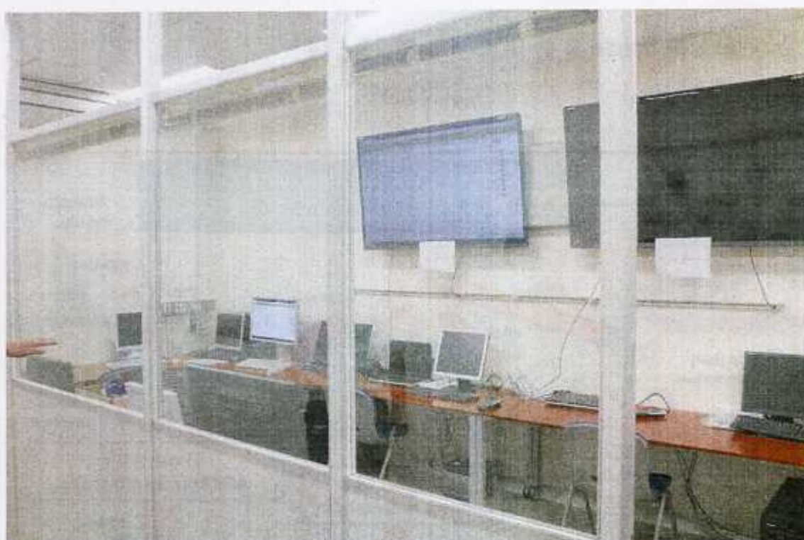
圖 14 Demand Response Automation Server Operation Room 實景
