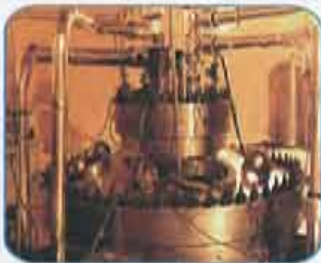
高通量工程试验堆顶盖 Top Head of High Flux Engineering Test Reactor
