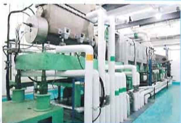
200吨铀/年干法转换系统研制 Development of 200tU/a IDR conversion system
