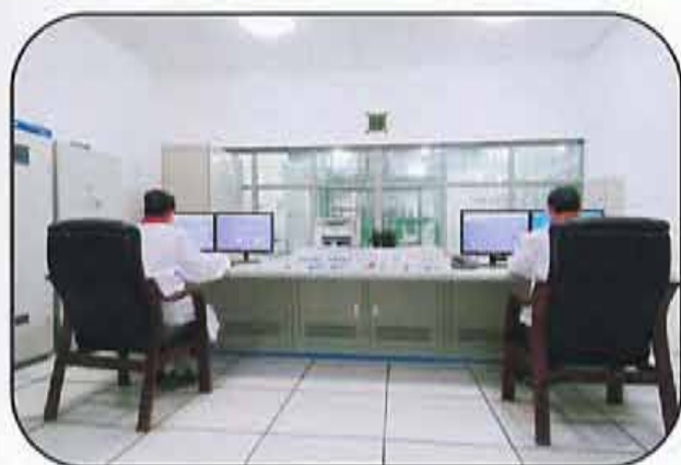
控制室/Control room
