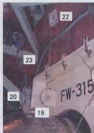
Around Feed-water pipe
