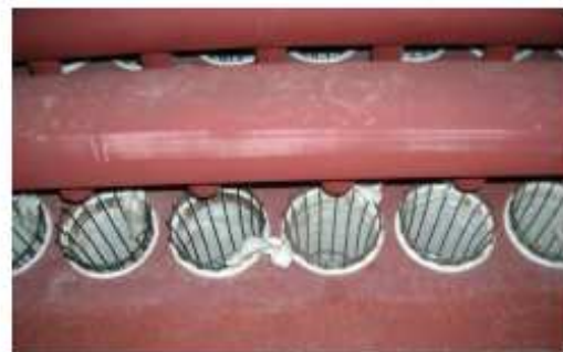
Top of filter bags in tubesheet Nozzle pipe above bags
