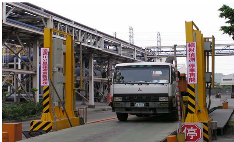
Figure 7. Portal type radiation detector in a steel mill
