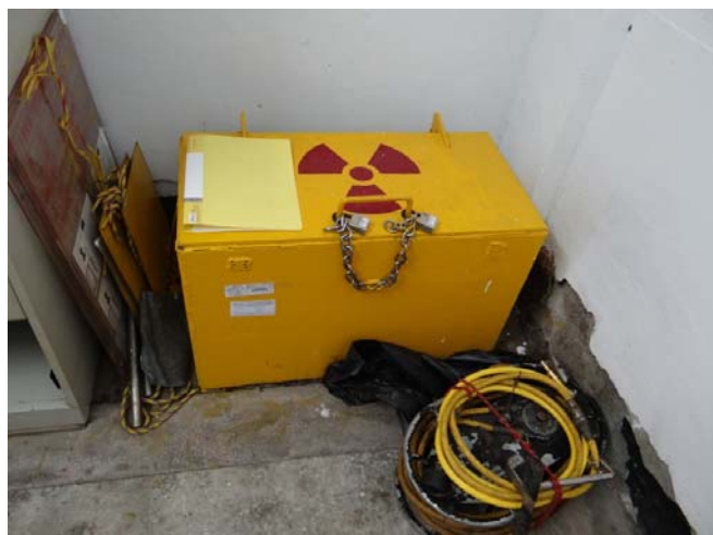
Figure 3. Delay system – locked-up storage cabinet dedicated for radioactive sources
