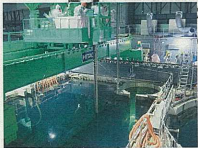
Removal of the fuel from Unit 4 Spent Fuel Pool has started on November 18.
