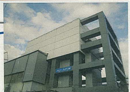
Reactor 4 with external walls and ceiling panels installed. A structure to support the fuel taking facility is installed so that the work can be carried out without applying the weight of the facility onto the reactor building.
