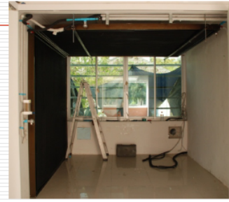
Roof with radiant cooling
