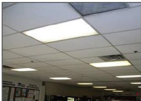
original system was 3-lamp T8/T12 fixtures with switches
