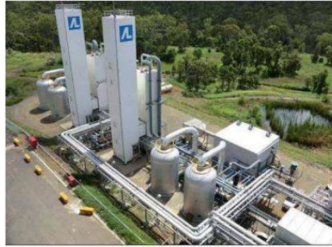
Air Separation Unit (ASU)
