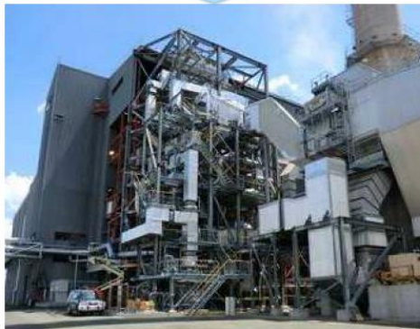
Boiler (After modification)
