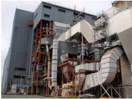
Boiler (Before modification)
