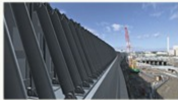
Image of tsunami protection wall
