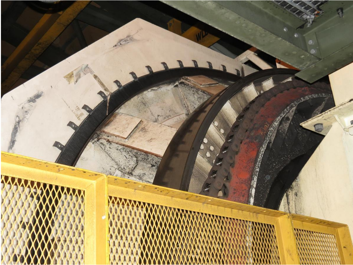
圖34 Narrabri 碎煤廠房 Rotary Breaker
