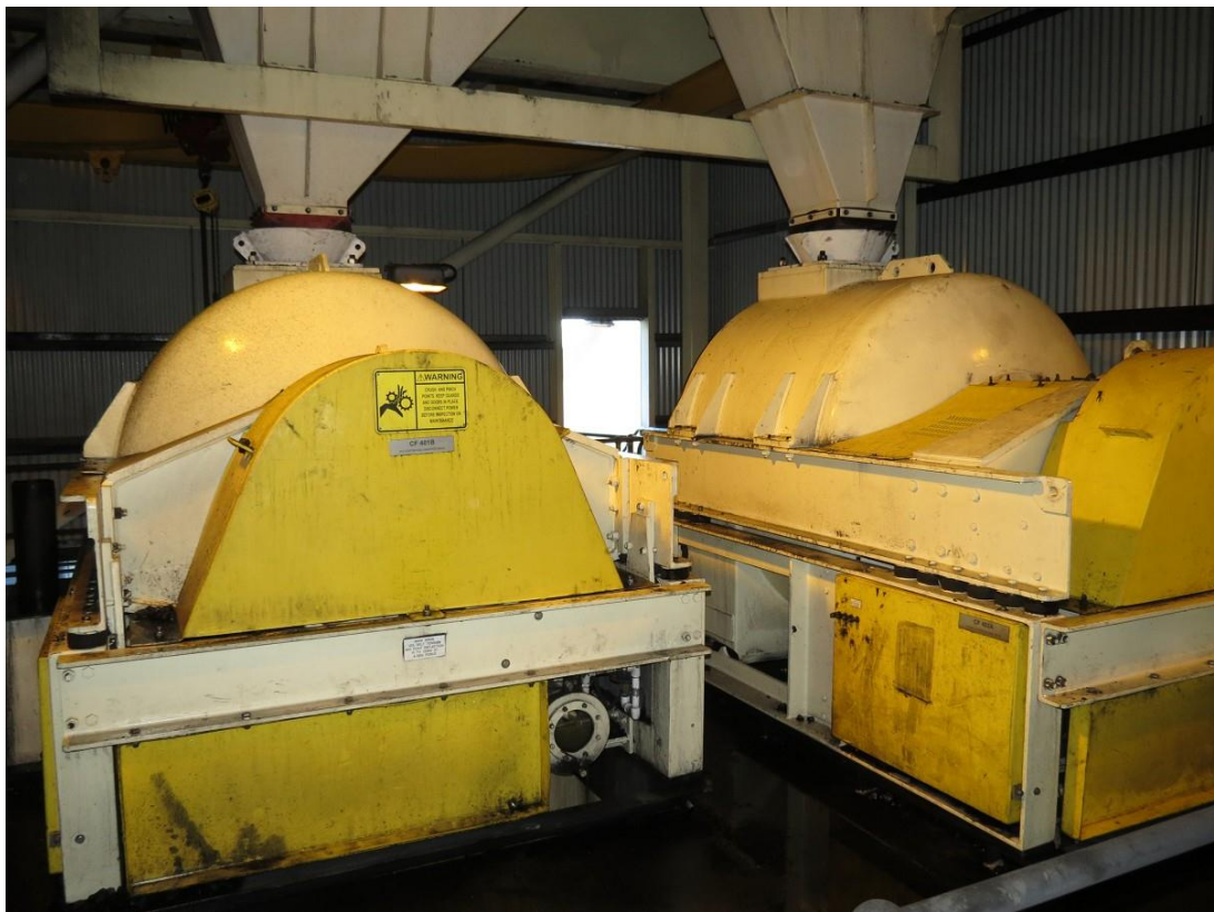
圖43 Narrabri煤礦CHPP Centrifuge (PCI & Thermal Coal)
