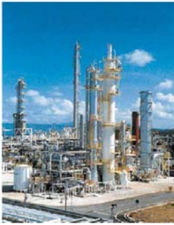
Figure 3.5 CO 2 capture plant in Malaysia using a 200 tonne d -1 KEPCO/MHI chemical solvent process (Courtesy of Mitsubishi)
