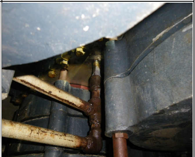
Water Detector Pipe and High Voltage Bushings 檢漏
