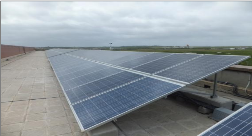
Solar panels at the Jianshan Power Plant
