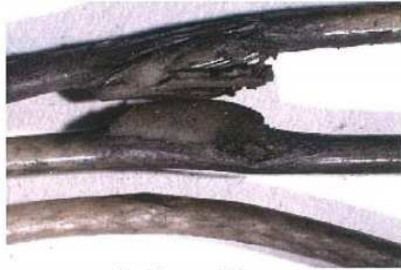
Heat Damaged Wires
