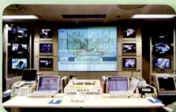
BHS control room
