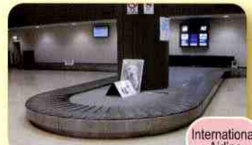
Baggage claim conveyor
