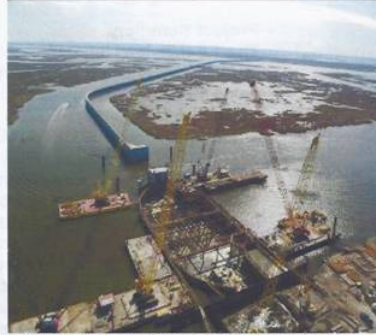
The GIWW sector gate and barge gate
