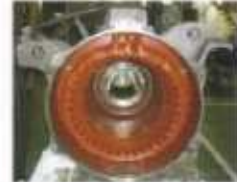
Inside motor after two years of operation
