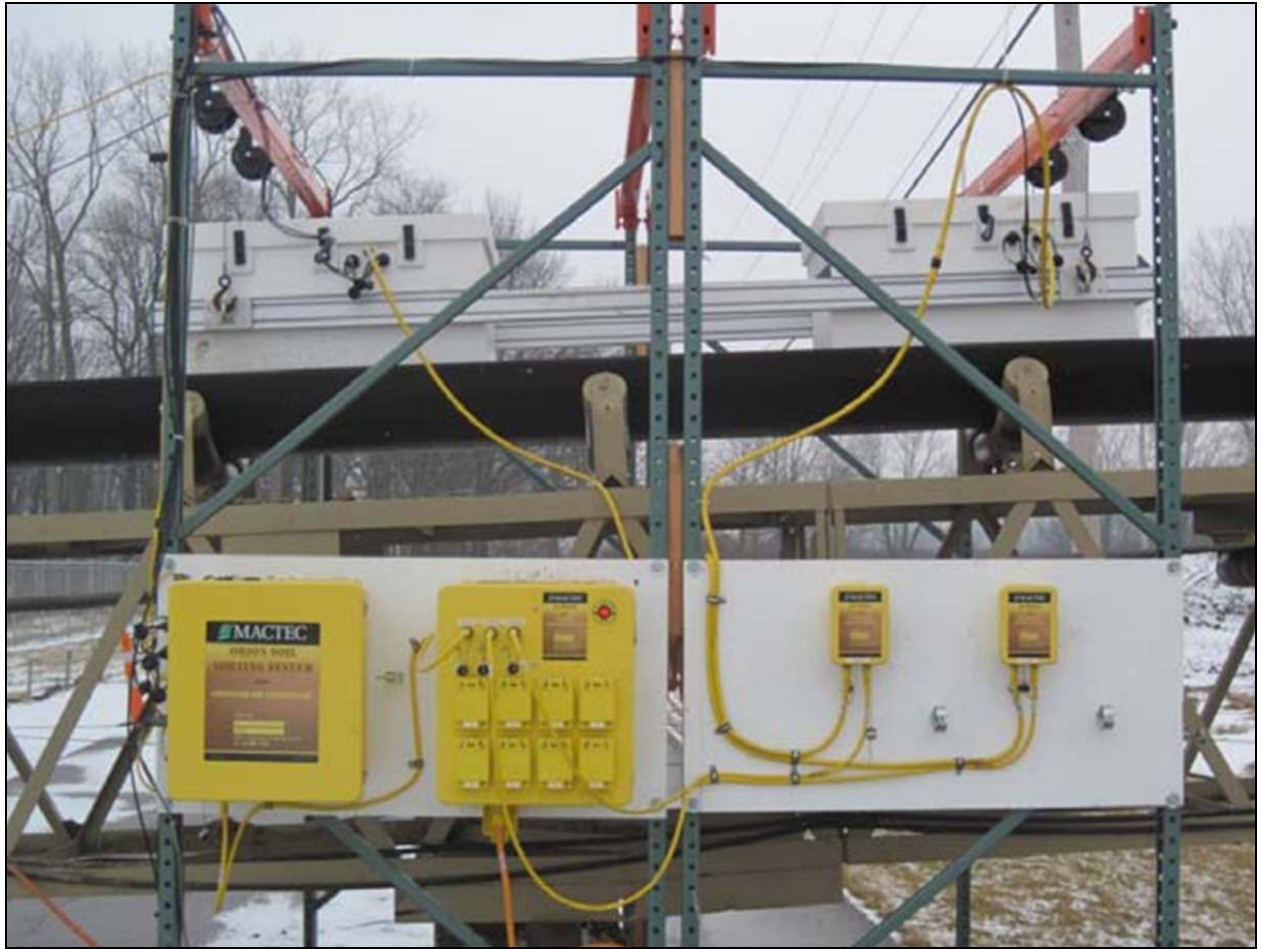
Figure 4 Auxiliary QA/QC Detection System Mounted on Conveyor #6
