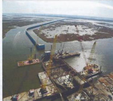
The GIWW sector gate and barge gate
