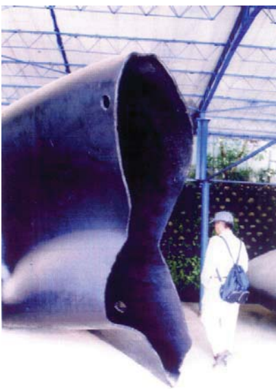
Fig. 2 Damage to a 2600 mm Pipe in the 921 Chi-Chi earthquake
