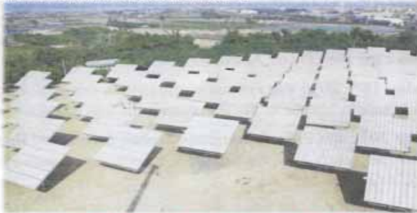
1 MW On-Grid HCPV Demonstration Plant
