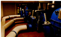
Pipe dreams: deep down in the basement of a new apartment block, the waste is held in these vacuum vessels. Each can be emptied automatically from the truck cab in the right sequence.
