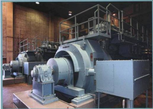
The Power Generation Station recovers most of the available energy from methane gas to produce electrical power needed for wastewater treatment.
