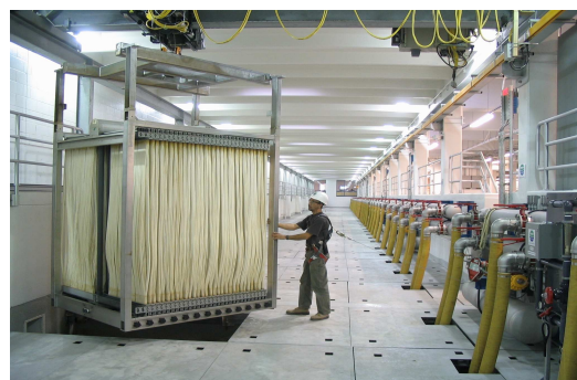
THORNTON 40 MGD ZW 500 SYSTEM
