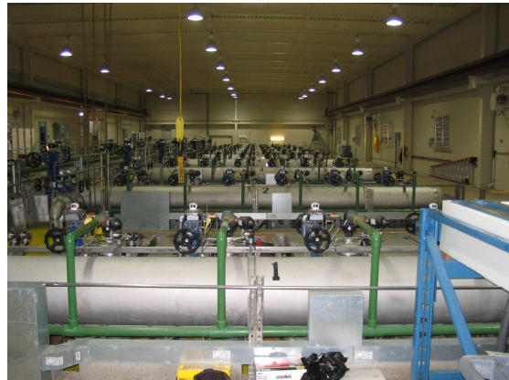
40 MGD SSJID ZW 1000 System (Covered Tanks)
