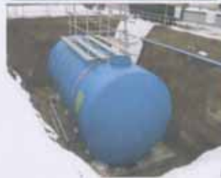
Fire protection water tank
