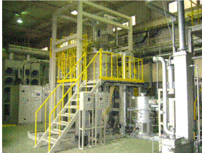
Fig.3. Exterior view of the demonstration scale UHFIF
