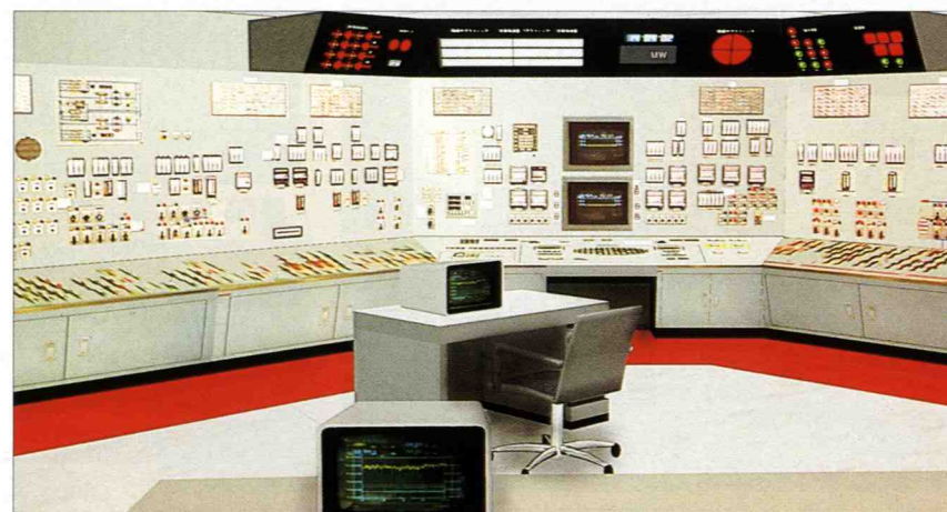
Further Improvement of Main Control Room Function
