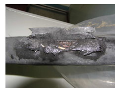
Failed Wet Cable
