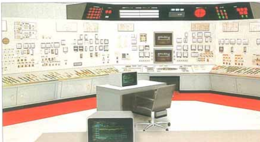
Further Improvement of Main Control Room Function
