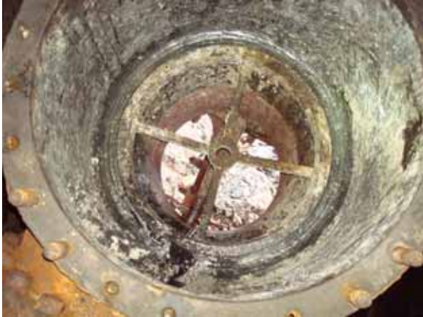
OVERBOARD SEA VALVE 檢查
