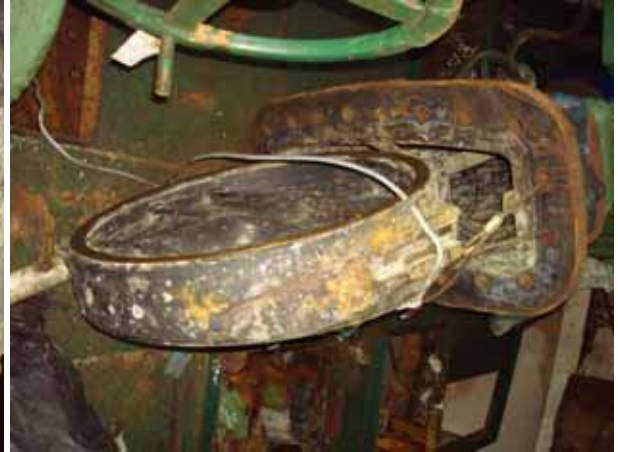
OVERBOARD SEA VALVE 檢查
