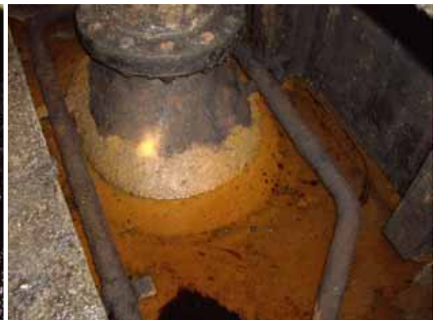
6P stripping bellmouth underside
