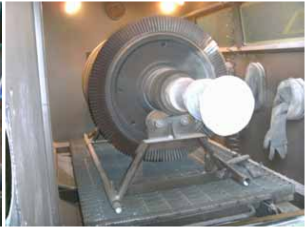
CARGO PUMP TURBINE ROTOR
