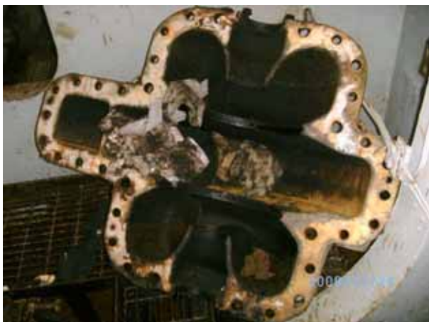
Cargo pump casing
