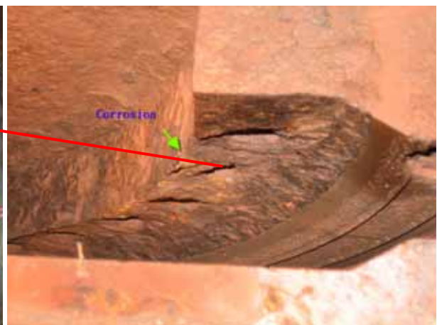
Heavy corrosion for nozzle &amp; bolts
