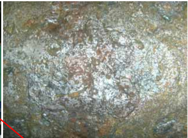
Heavy corrosion on surface
