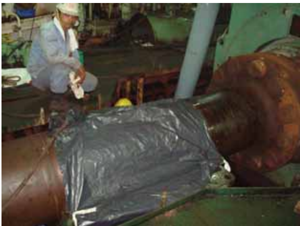
Intermediate shaft bearing dismantled
