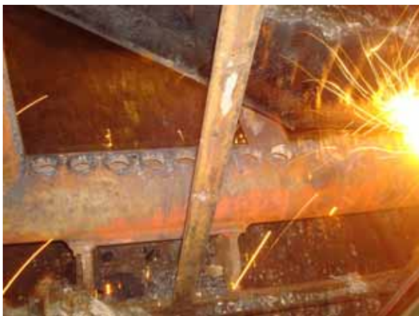
Rear wall Tube cutting
