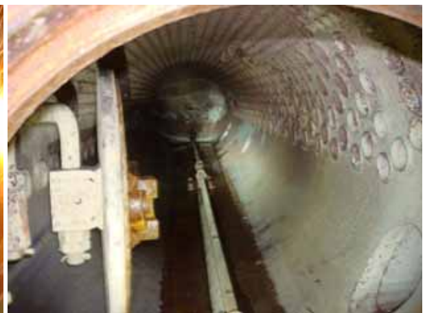
Boiler Water Drum
