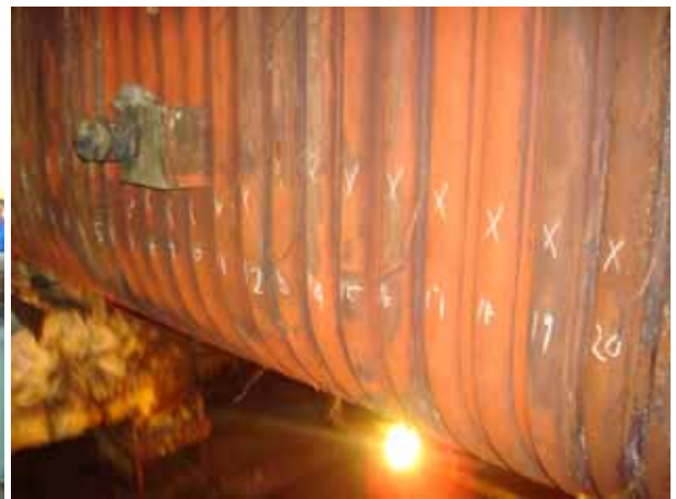
Boiler Furnace wall tube
