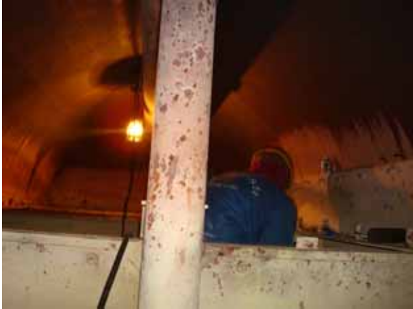
Boiler Steam Drum
