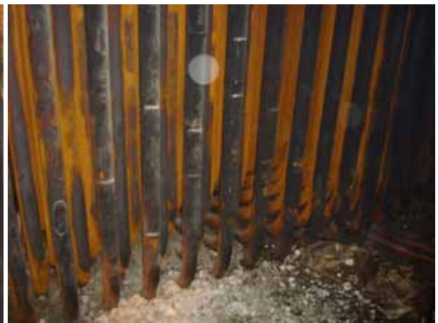
Screen tube underside condition worse
