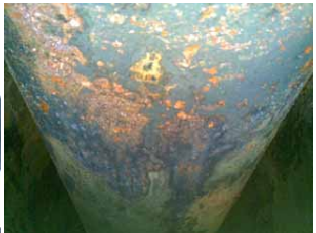
Inside of the PV breaker
