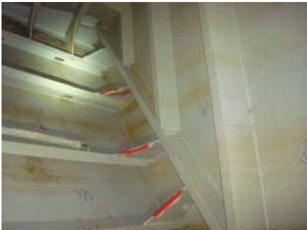
Bracket heavy corrosion
