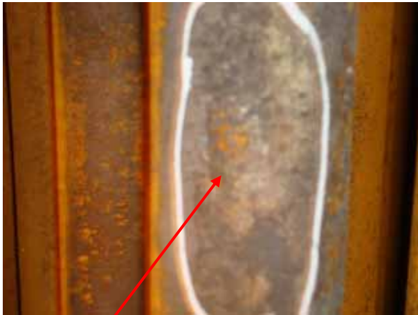
Screen tube pitting hole
