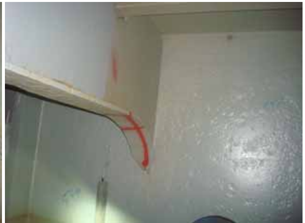
Face plate heavy corrosion
