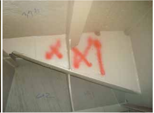
Bracket heavy corrosion
