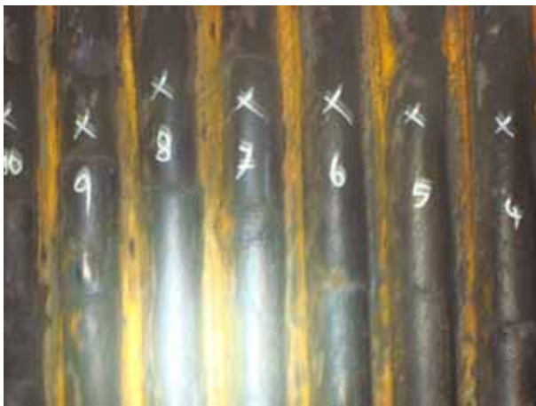
Furnace side Wall tube
