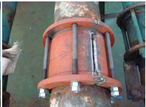
Expansion joint for cable pipe
