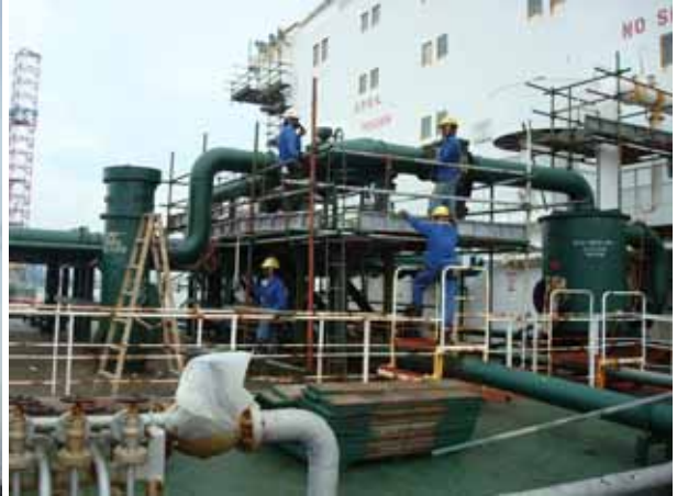
STAGING FOR IG VALVE
