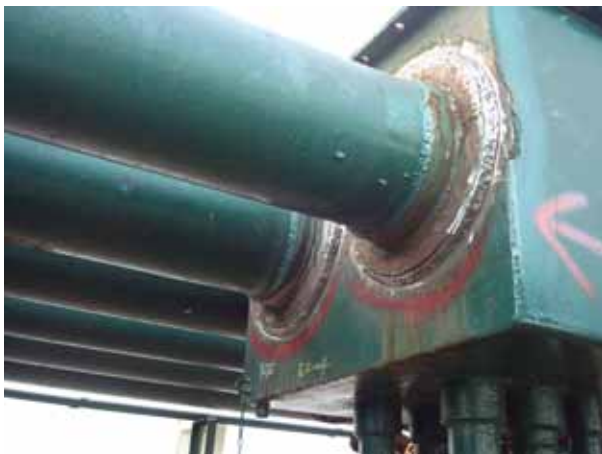
Junction box for cable pip
