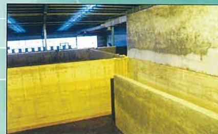
垃圾滲瀝液處理系統 Leachate Treatment System
