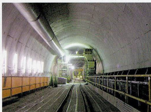
⑨千駄ヶ谷工区 継手：セグメント間—スライドロック/リング間—TA-SRING Joints : Between segments—Slide lock / Between rings—TA-SRING
