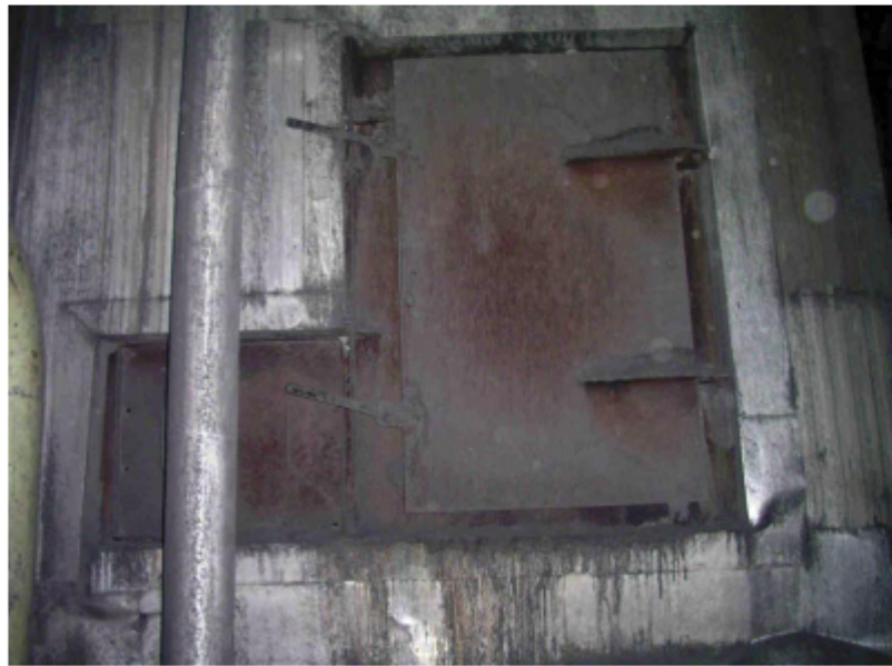
Furnace hopper front deadspace A side doors.
