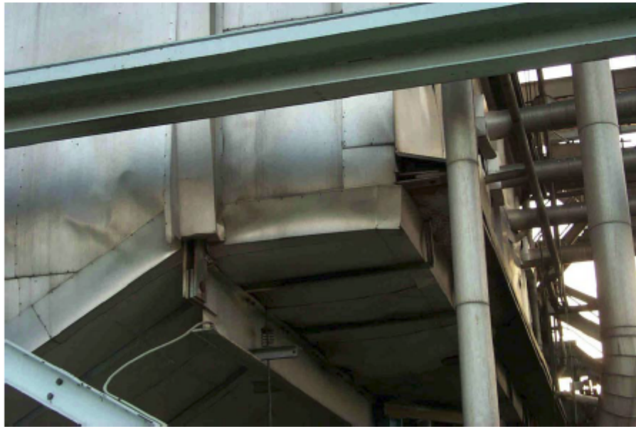
圖 2.2.1-10：案例 10 Casing leakage：Internal inspection found corresponding cracking of ductwork
