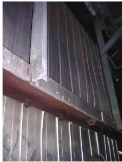
Furnace A side wall above Level 1. Normal hot spots at buckstay clips - no defects.
