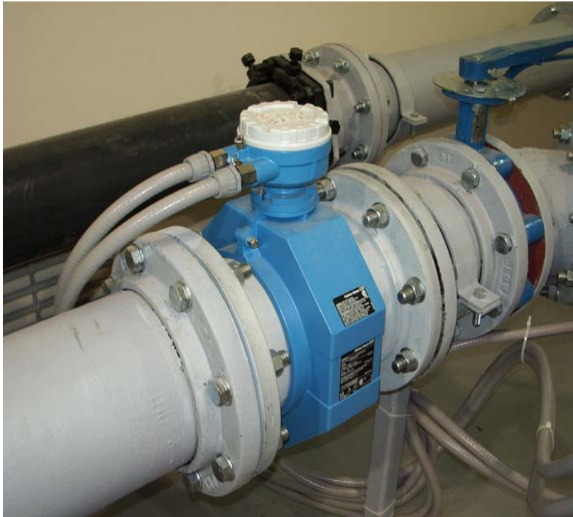
200 mm (8") Reference Electromagnetic Flowmeter (Fast Flow Tests) Coulter Meter Service
