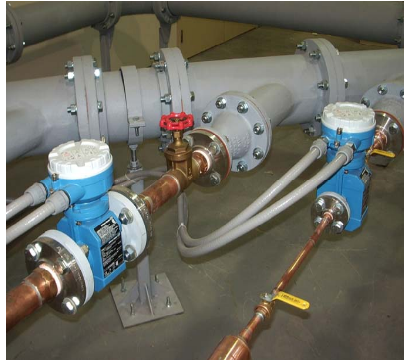
50 mm (2") & 13 mm (1/2") Reference Electromagnetic Flowmeter (Intermediate and Slow Flow Tests) Coulter Meter Service
