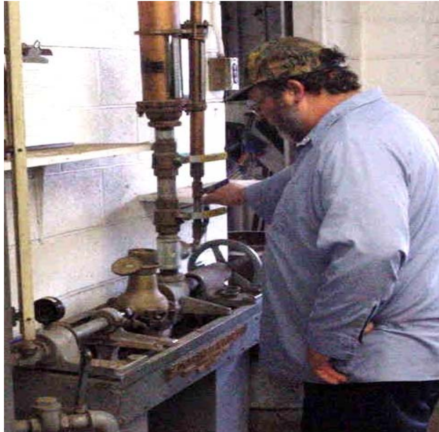
Small Meter Test Bench City of Brandon Canada
