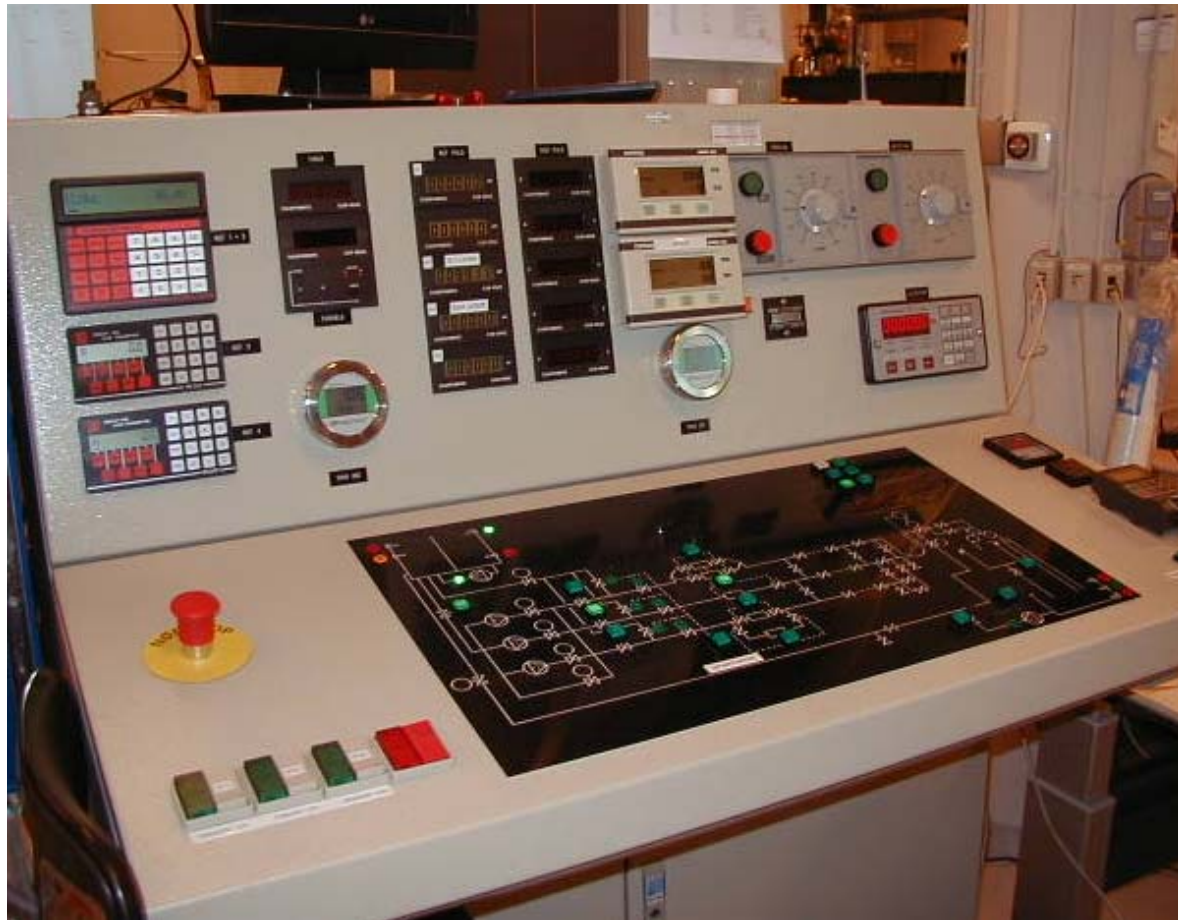
Test Bench Console Force Technology Denmark
