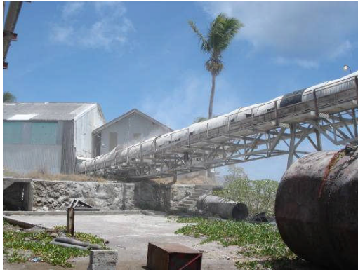
Figure 3 Photo Shore Bin & Conveyor
