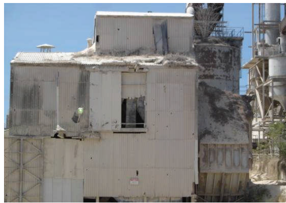
Figure 9 Photo South of Crusher Missing Sheets
