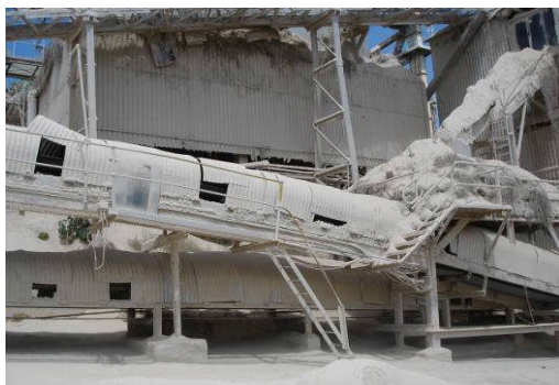
Figure 10 Photo Overflows at Crusher, CV #D1
