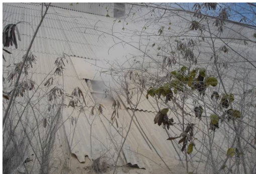
Figure 5 Photo Missing Sheeting Shore Bin
