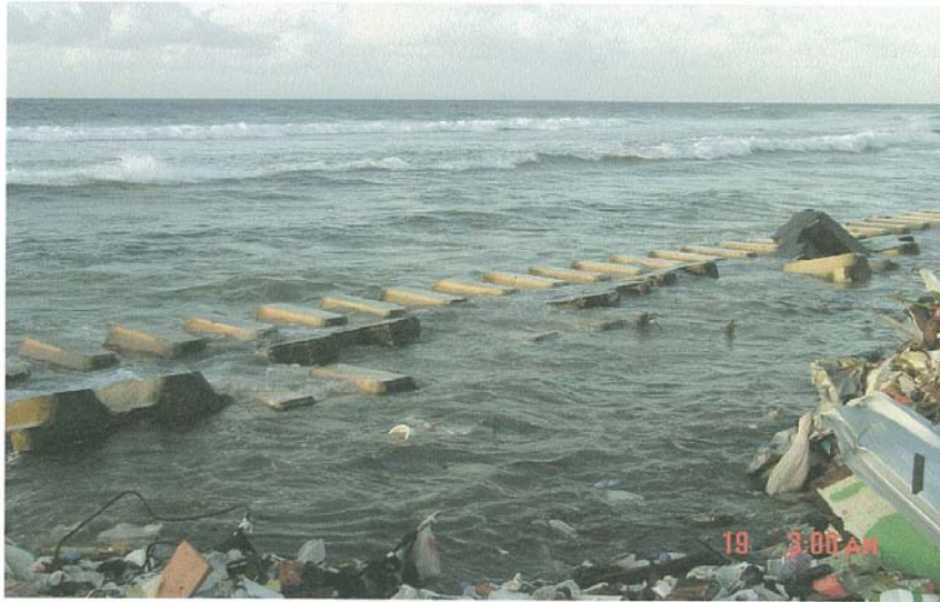
SEAWALL FAILURE APRIL 19, 2007. HIGH TIDES AND A SOUTHERLY WIND CREATED 2'-3' WAVES THAT CAUSED THE WALL TO FAIL
