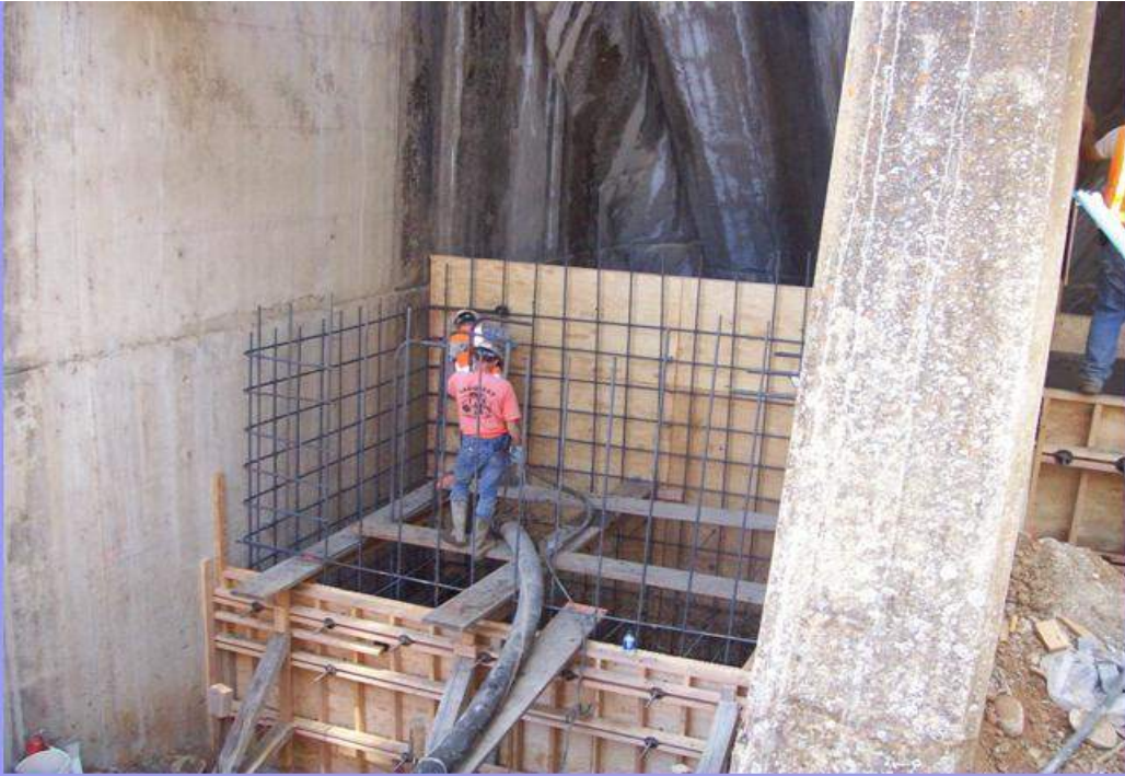
The 10' wide starter wall in the bay between 18-19 will be placed in two lifts. The height of the first lift was 7' from the lowest point.
