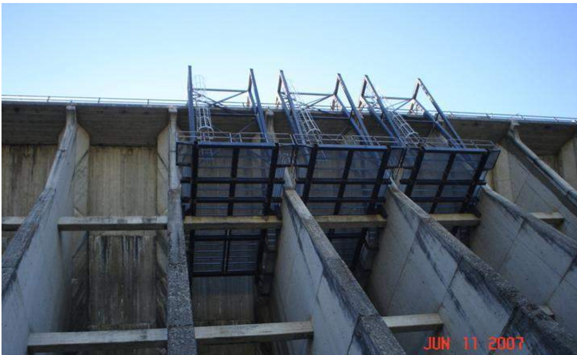
Three of the seven completed C-hanger setting in place on top of the dam
