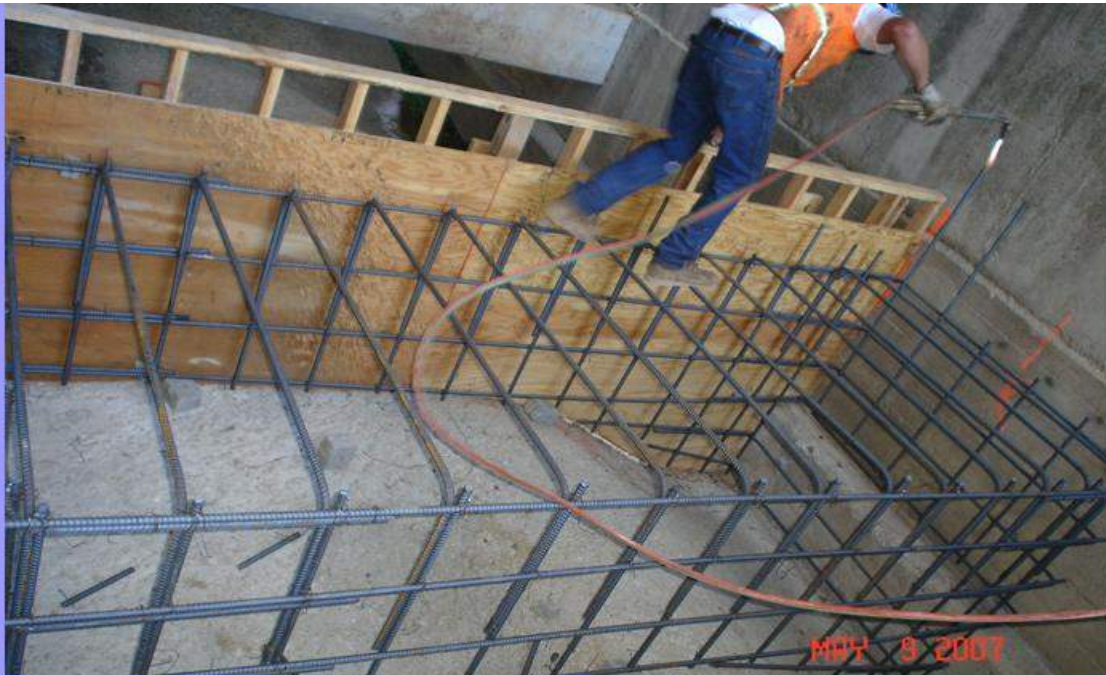
A truck load of rebar for the diaphragm starter wall was delivered. The iron workers installed the rebar in the bays between buttresses #37 to #42.
