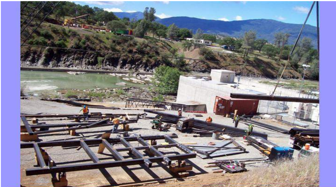
A crew fabricates the elevated access platform (C-hanger) . The approximately 16,000 pound C-hanger will be supported from the top of the dam and provide access to construct the diaphragm wall, the capitals/struts, and the additional struts. There will be total of six C-hangers used in adjacent bays.
