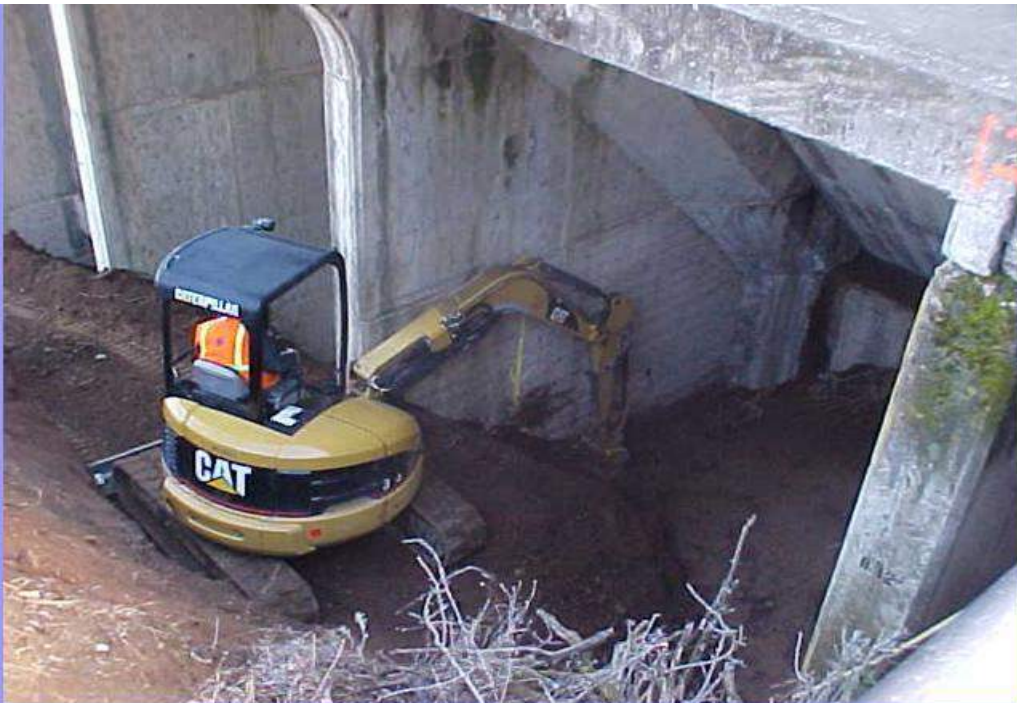
A small caterpillar excavator is used to establish access to and foundation cleanup in the bays between the buttresses.
