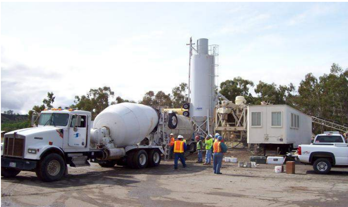
The contractor's portable batch plant was operational on May 4. MPCO provided three 4,000 psi concrete mixes for test batches with 35% to 25% flyash.
