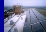
Diwan College, Tainan County Solar Thermal Water Heater System Installation area: 307.5m 2 (for 450 students)
