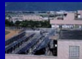
Hualien College, Hualien County Solar Thermal Water Heater System Installation area: 77m 2 (for 115 students)
